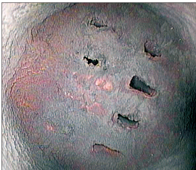
Figure 1: Water chamber with severely plugged ends of the hollow conductors.
