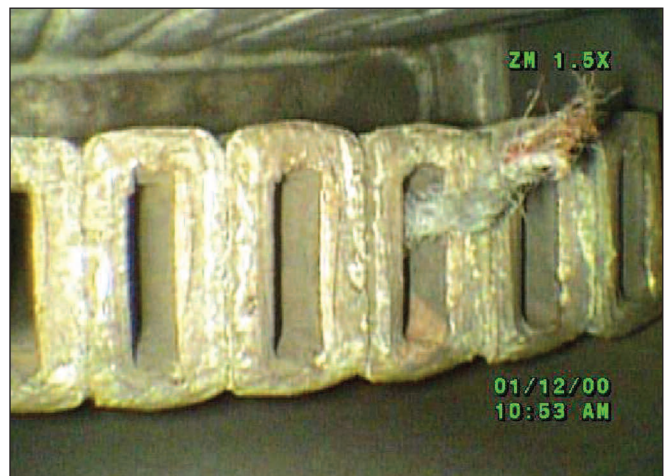
Figure 9: Hollow conductors with debris.
