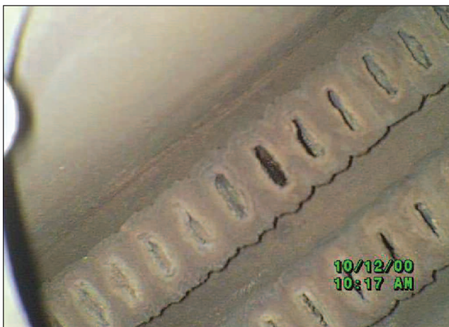
Figure 8: Hollow conductors with oxide plugging.
