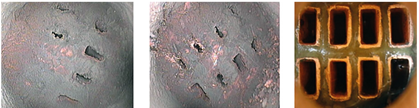
Figure 1: Plant O3. Water box before (left) and after (middle) mechanical cleaning. Right: after subsequent complexant cleaning [10]. Note that all photos were taken from the same water chamber.
