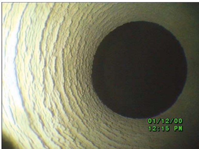
Figure 8: Heavy copper oxide deposits inside an insulating hose supplying water to a stator bar. These deposits were analysed as being mostly \text{Cu}_2\text{O} .
