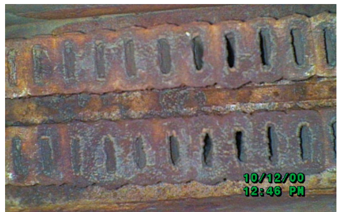
Figure 7: Stator bar inlet water box with copper oxide deposits as found during visual inspections at plant S. The areas around the hollow conductor inlets are particularly affected, as they lie in an area of high turbulence and flow velocities.
