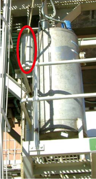
Figure 9: Head tank and expansion vessel for the stator water detrainment tank vent line. The expansion vessel is the small vessel to the left of the larger head tank. It prevents the standing water in the line from escaping through the vent if large amounts of gas are released at once.
