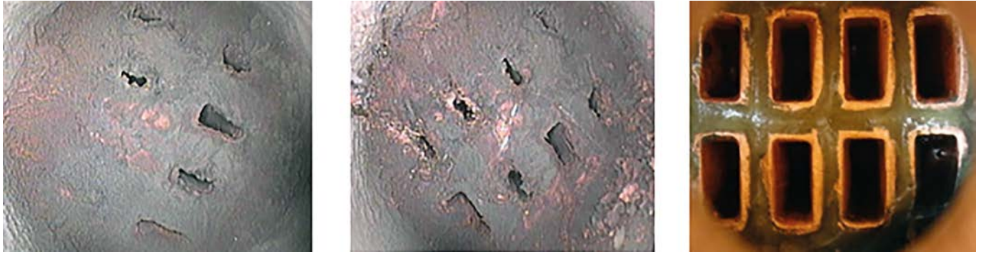
Figure 11: Stator bar inlet water box as found (left), after mechanical treatment with a metal rod to open flow passages (middle), and finally after targeted chemical cleaning (right) [10].
